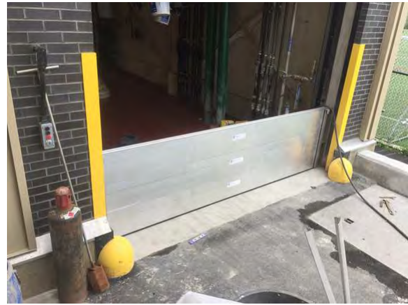
Figure 4 - Headworks Flood Barrier
